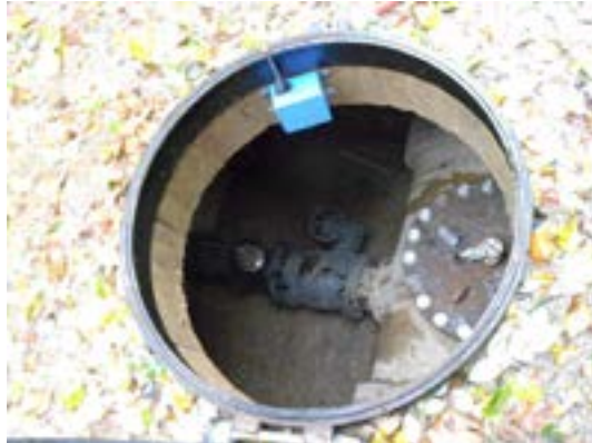
Fiber manhole sensor
